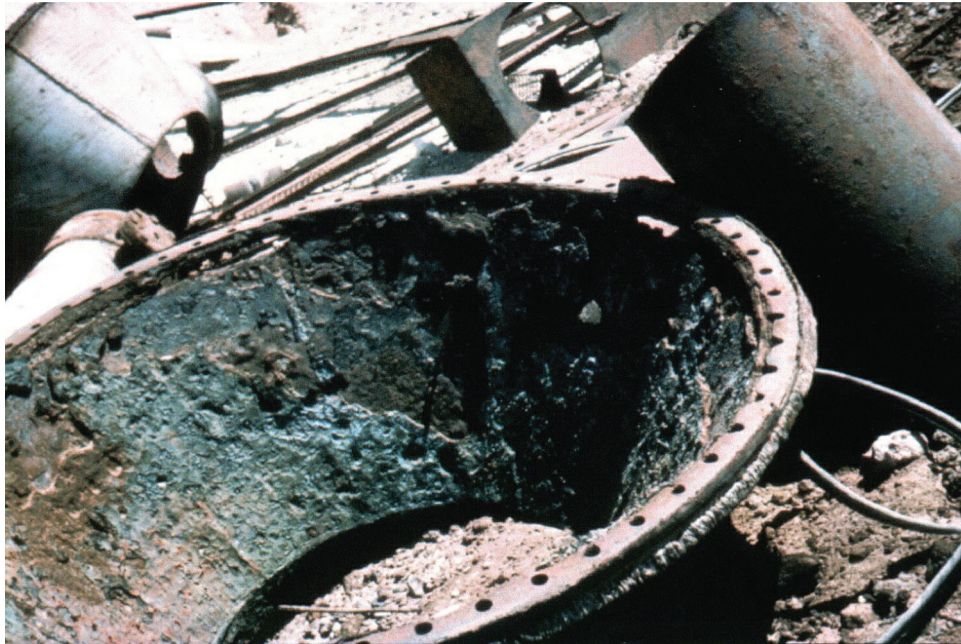
FIGURE 1.2: Excessive galvanic corrosion of a carbon steel water box from a multi-stage flash desalination plant.
